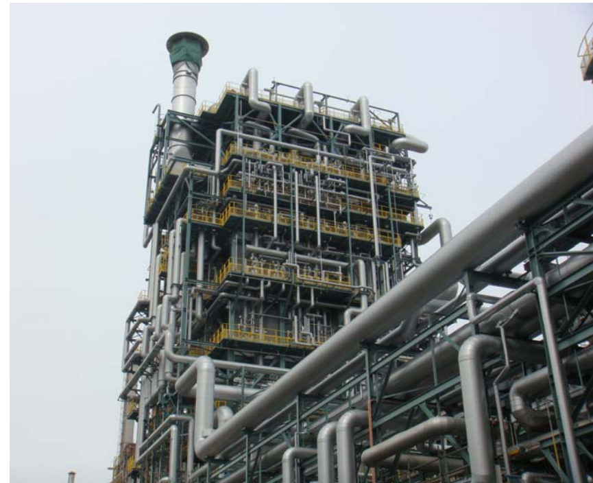
New cracking furnaces
